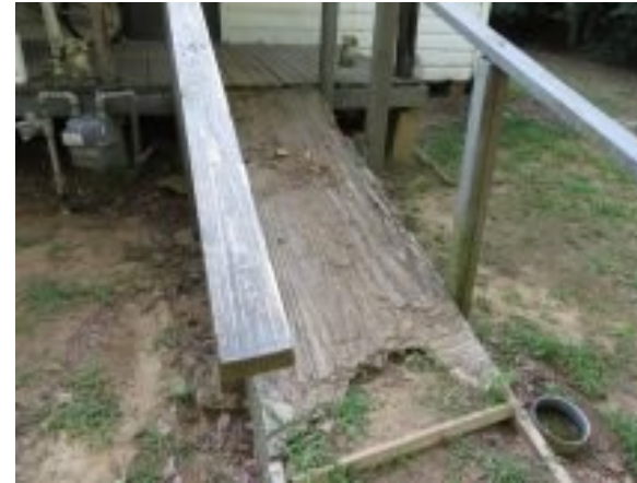
Dilapidated ramp in neighborhood
