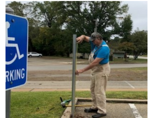
John installing new parking signs in our parking lot. Building & Grounds at work!
